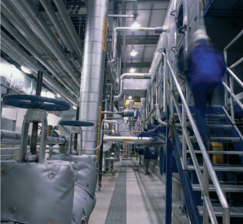
Plant control solutions
